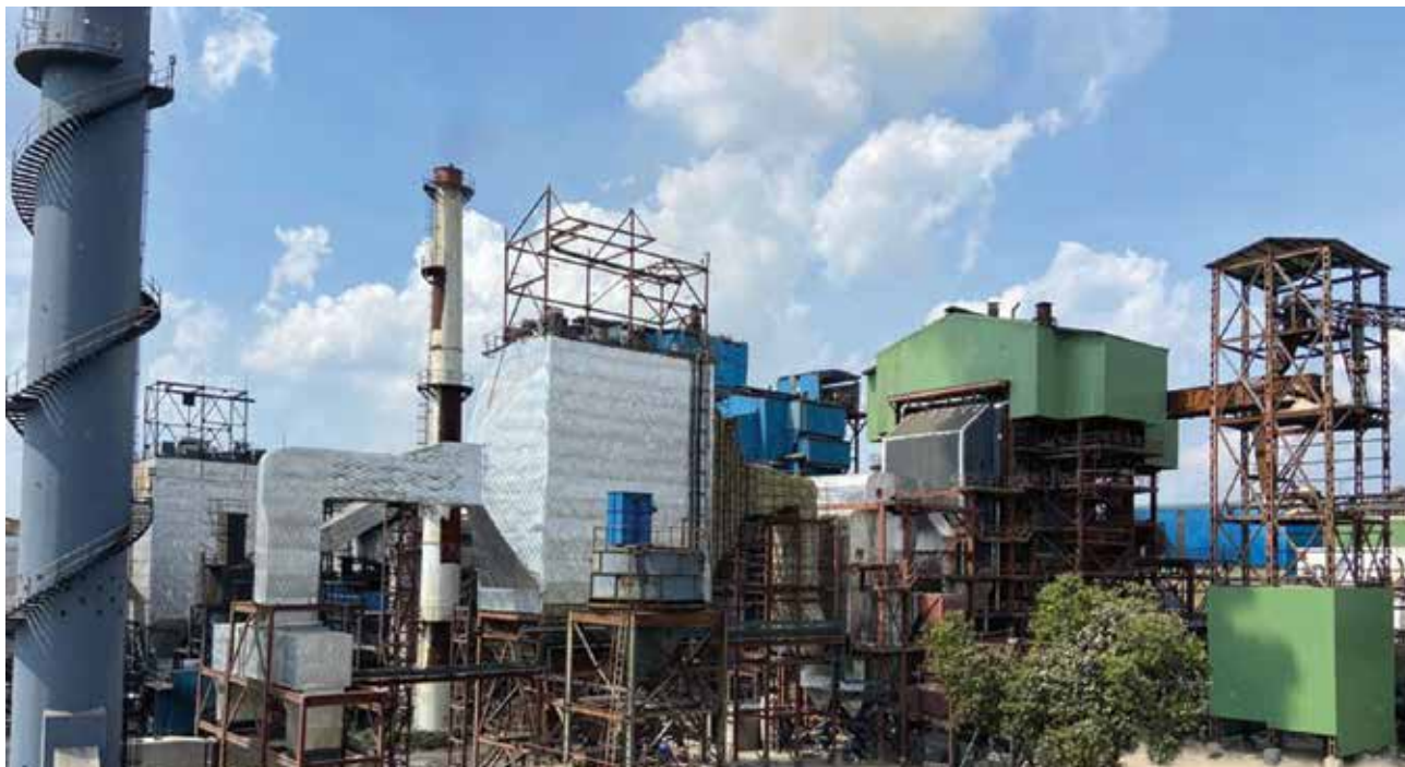
Cogeneration Plant at Haliyal
